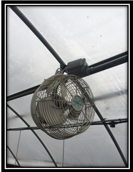
Two circulation fans
