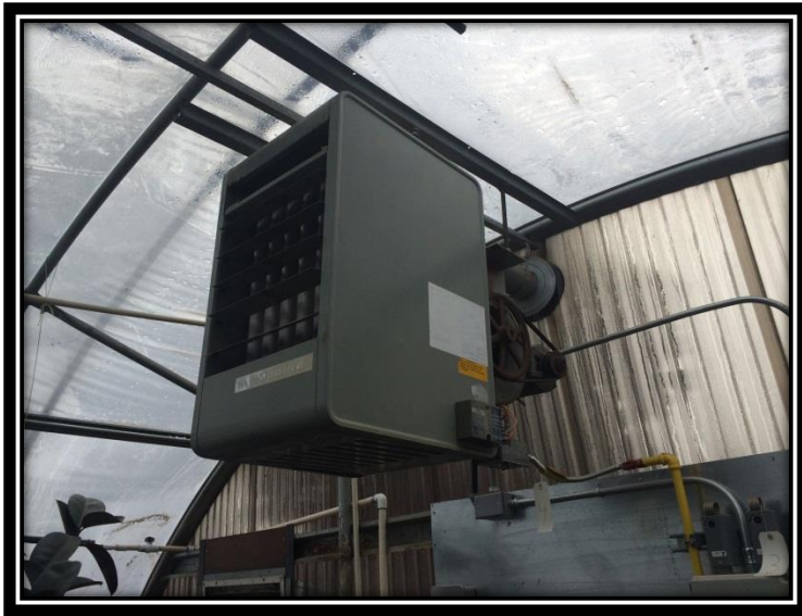
Heater was relocated to a safe location
