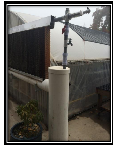
New water return and pump
